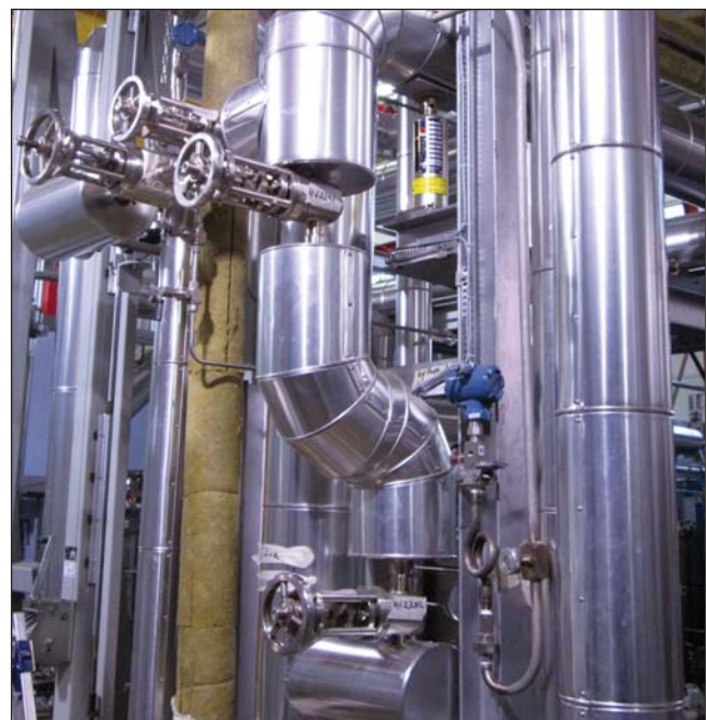
Forged pressure seal on site.
